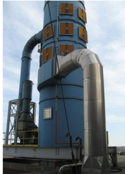
Baghouse operation and maintenance costs are largely a factor of the unit's design.
